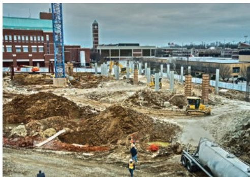
The new Belknap Academic Classroom Building is on schedule for a fall 2018 opening.
